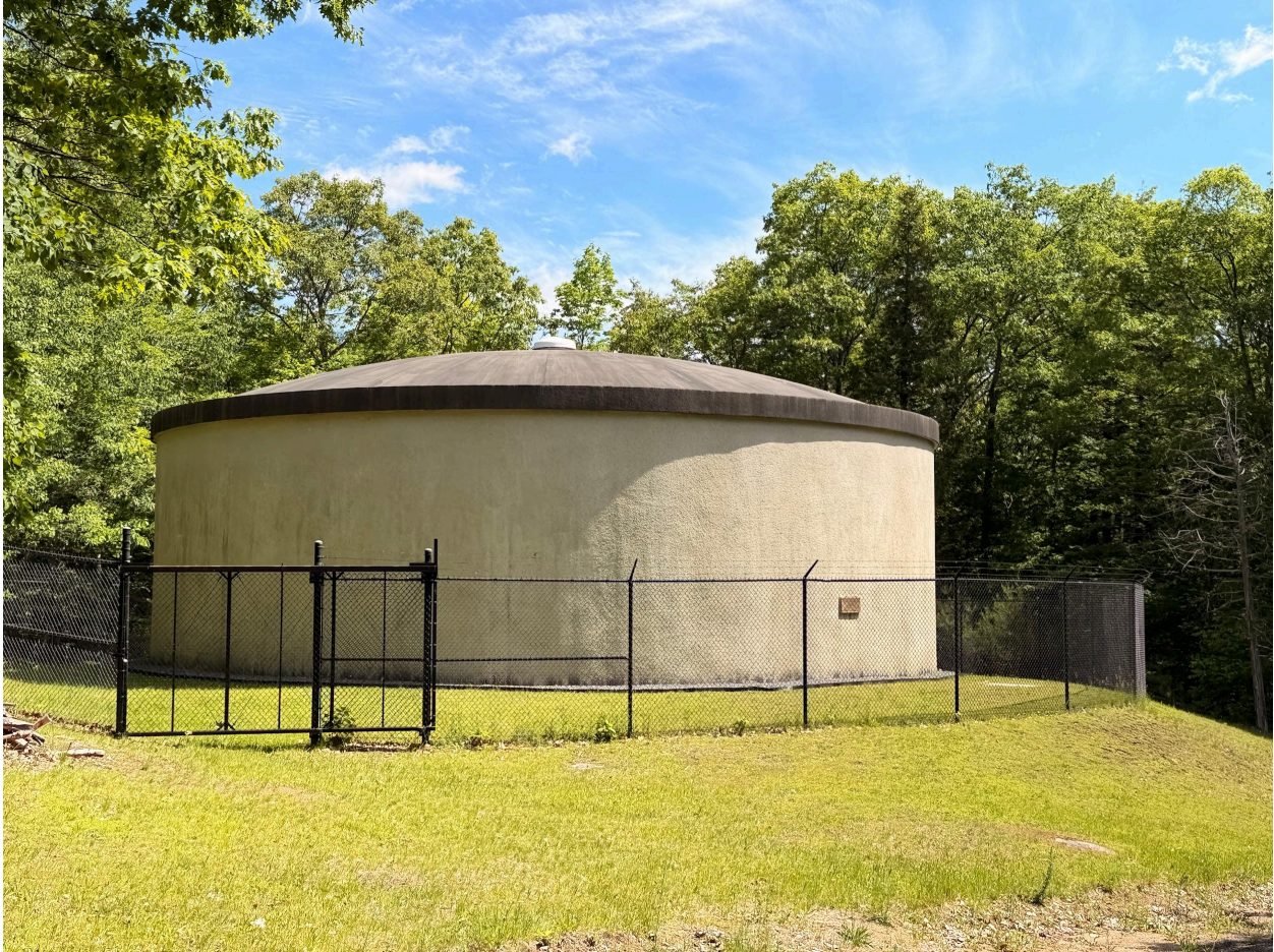
Clean water holding tank:
